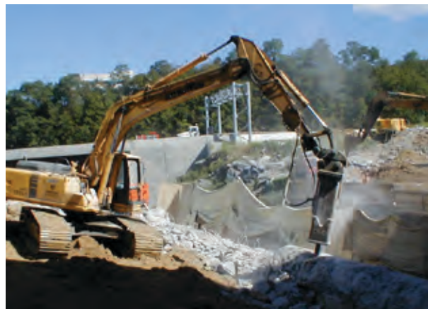
Excavator equipped with an enclosed cab and hoe-ram demolishing a concrete wall.
