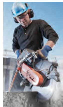
A worker cutting a concrete block using a handheld masonry saw with an integrated water delivery system.
