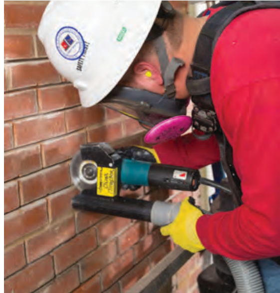
Worker grinding mortar from between bricks with a handheld grinder equipped with a shroud and dust collection system. In addition, worker is using respiratory protection.
