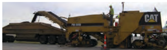
Milling machine milling asphalt road and loading debris into a haul truck.
