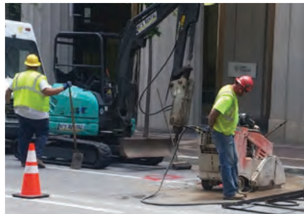
Worker using a walk-behind saw with an integrated water delivery system to cut asphalt roadway.
