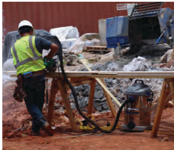
Worker cutting fiber-cement board outdoors using a handheld power saw and dust collection system. The dust collection system consists of the shroud on the saw, hose, and dust collector positioned between the saw horses.
